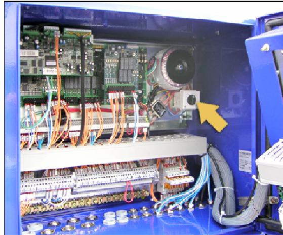
Fig. 26. Switch inside the cabinet
