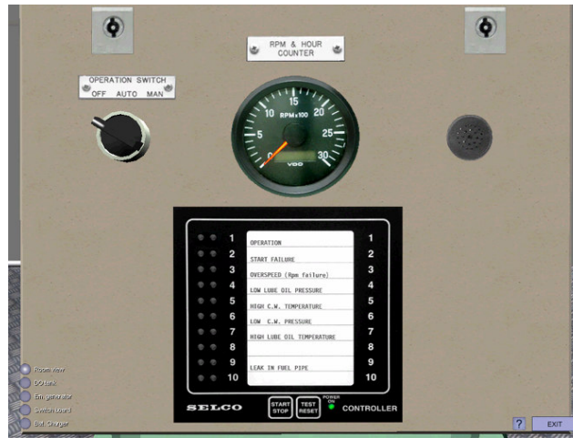
Fig. 6. SELCO control panel
